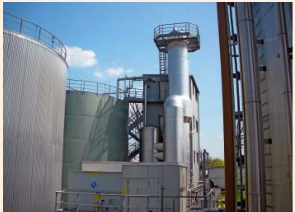
Product tank store and emulsion evaporation plant of Südöl Mineralöl Raffinerie GmbH in Eisingen, Germany
